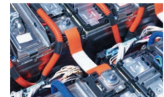
Connection resistance of battery busbars
